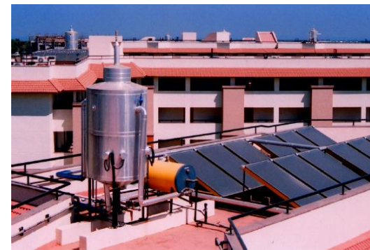
Systems installed at Infosys, Bangalore
