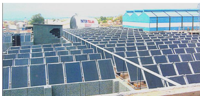
50,000 lpd systems at a Textile factory in Gurgaon Haryana through soft loan from Canara Bank
